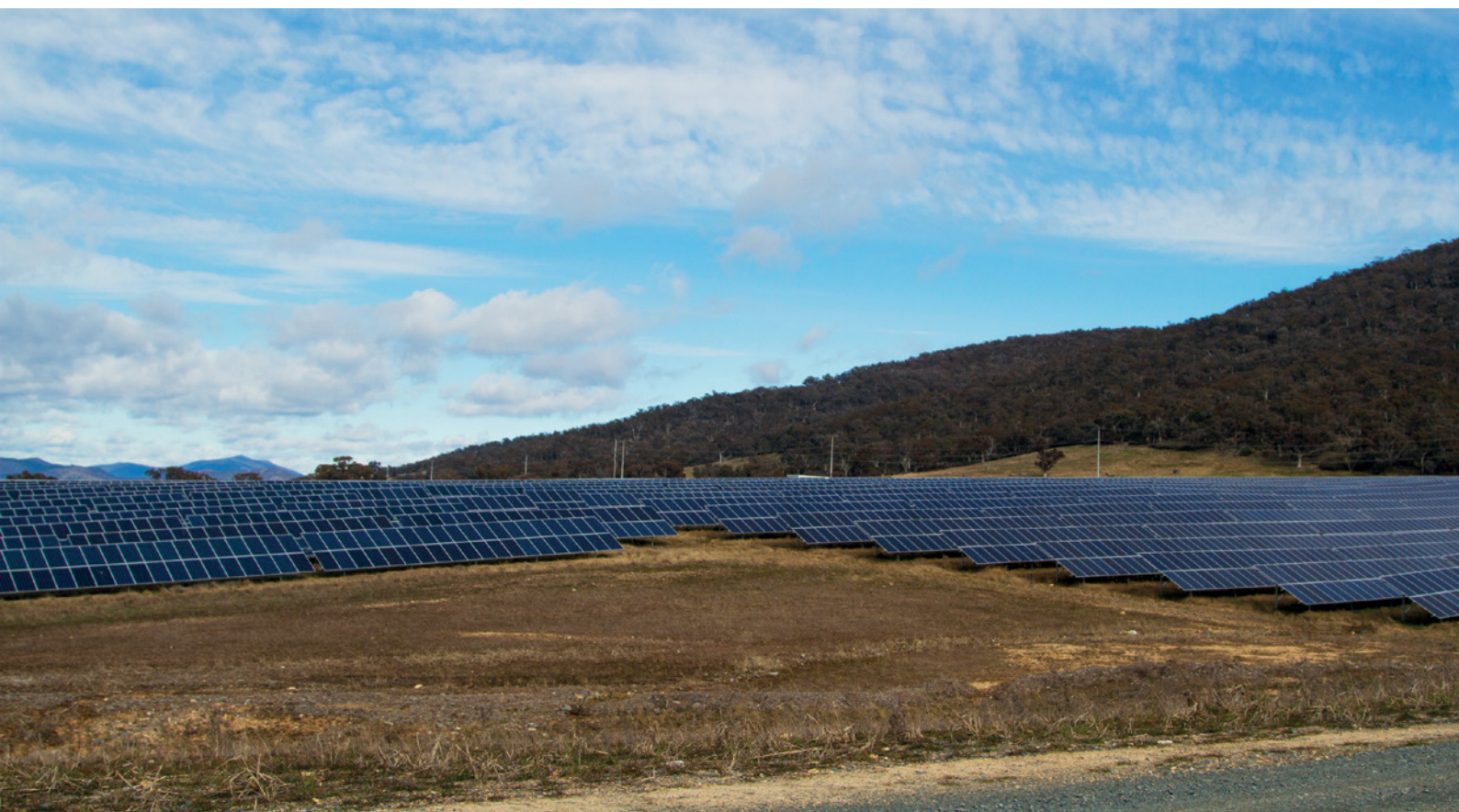
Figure 5: Royalla Solar Farm.
