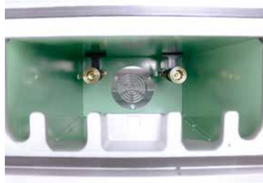
Convention Center Floor Box water and compressed air compartment.
